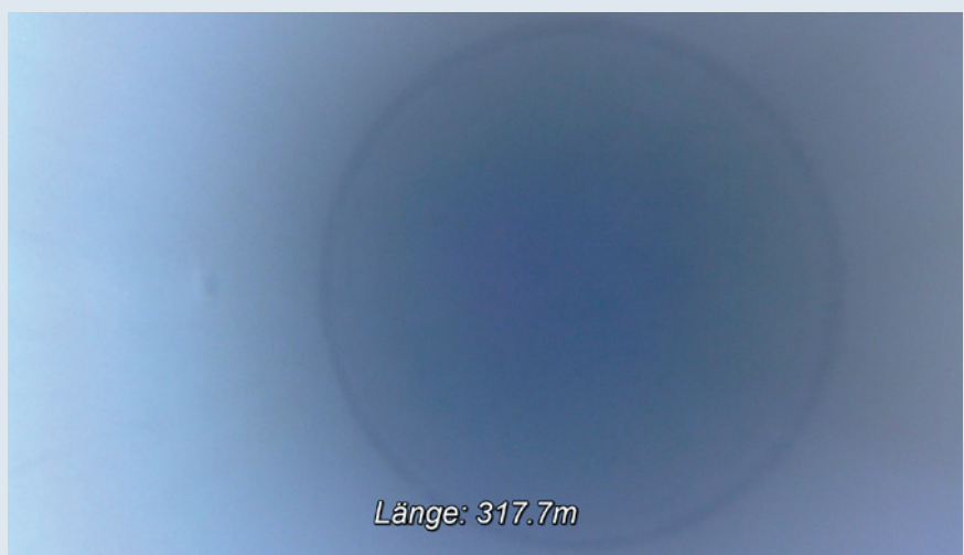
Figure 9: Video image pipe interior
